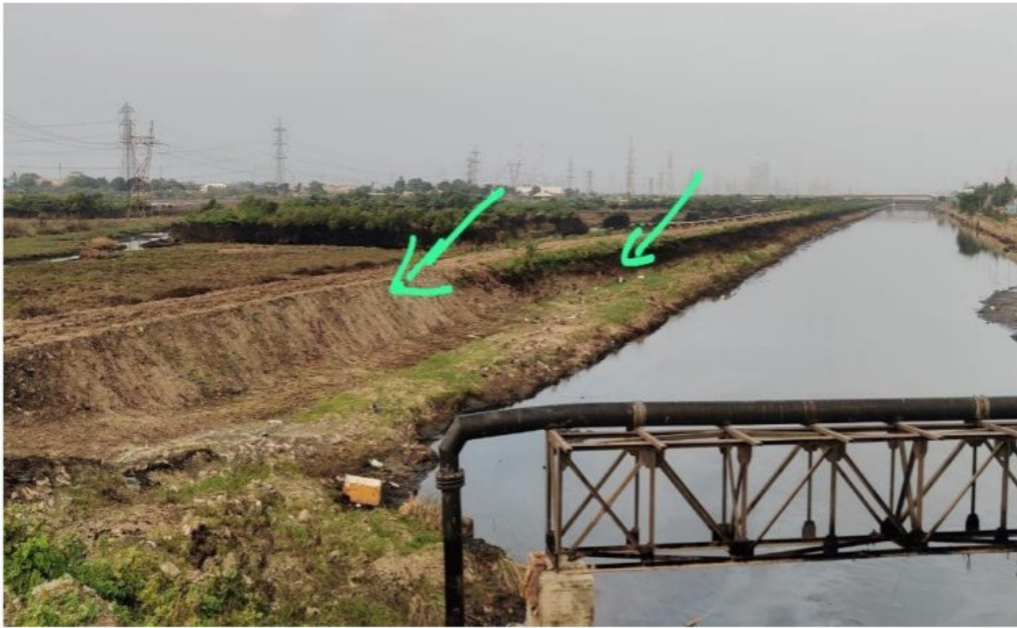
Figure 14: B canal possibly breached and oil stain covered.
